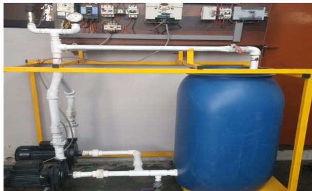
Figure 5. Pressure transmitter for water circulation framework.
